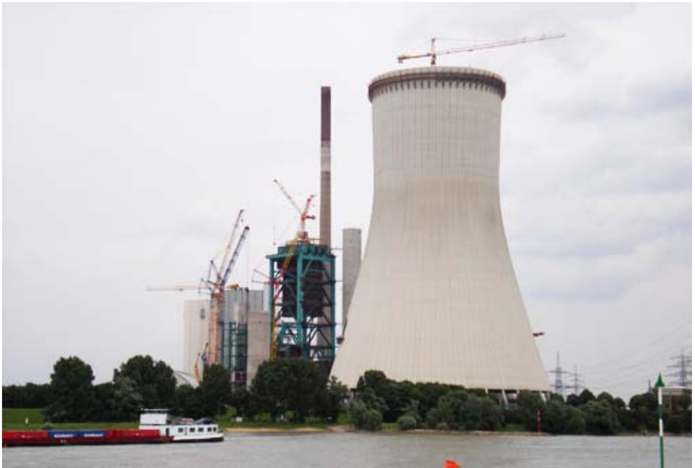
▲ The VSL Strand Lifting System has been used at Walsum Power Plant.
