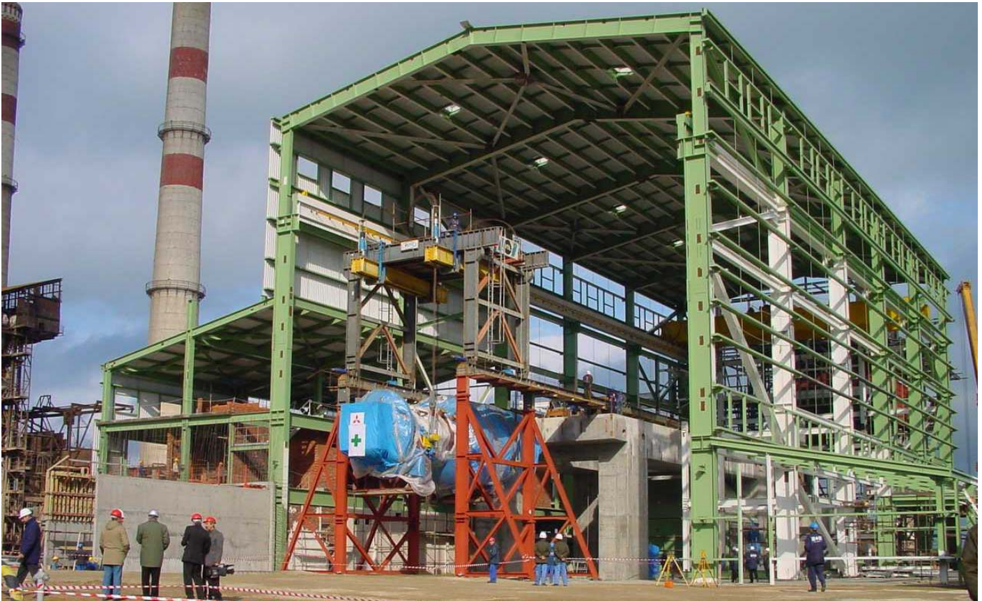
▲ View of the new machine hall with VSL lifting gantry and MHI Gas Turbine being lifted
