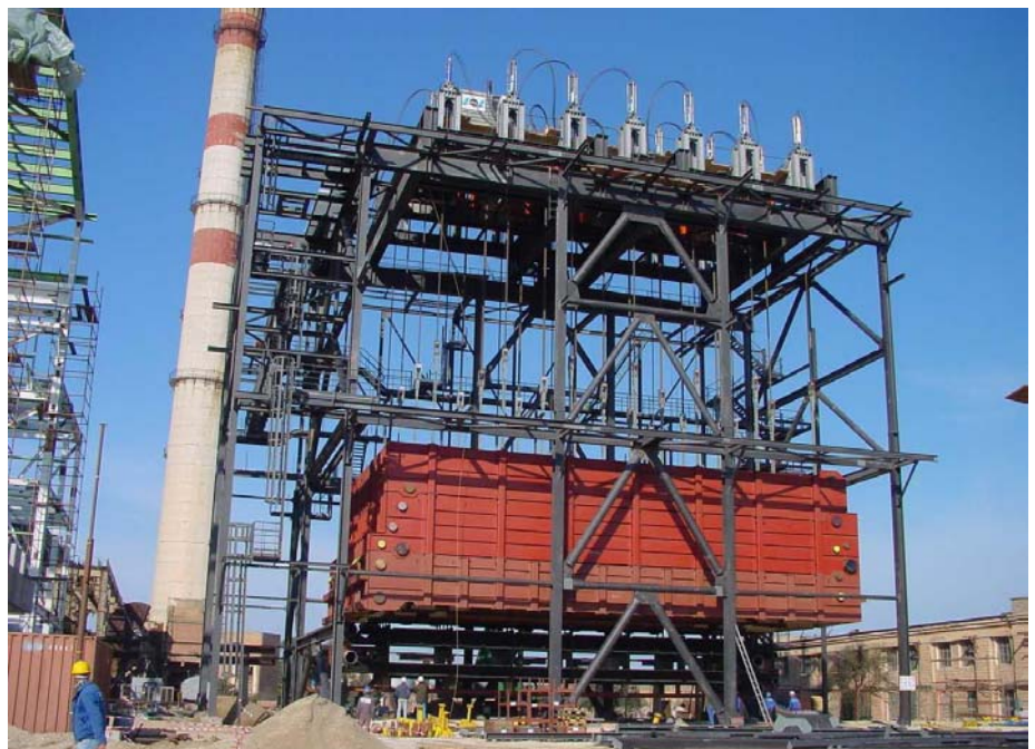
▲ View of boiler with 9 modules (3 levels) installed
