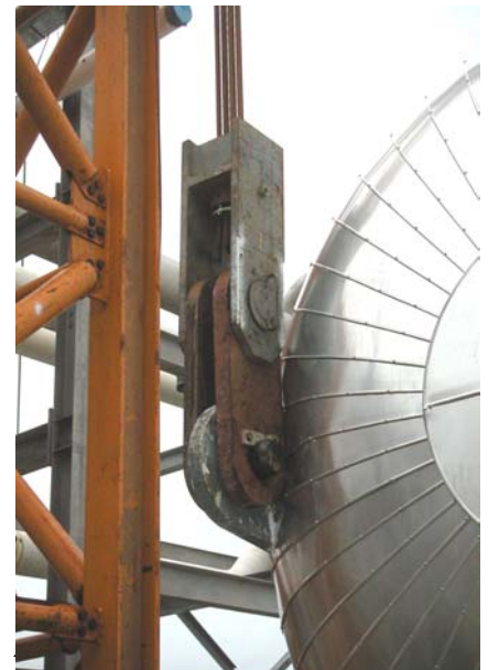
▲ Detail of lifting lug of deethanizer tower
