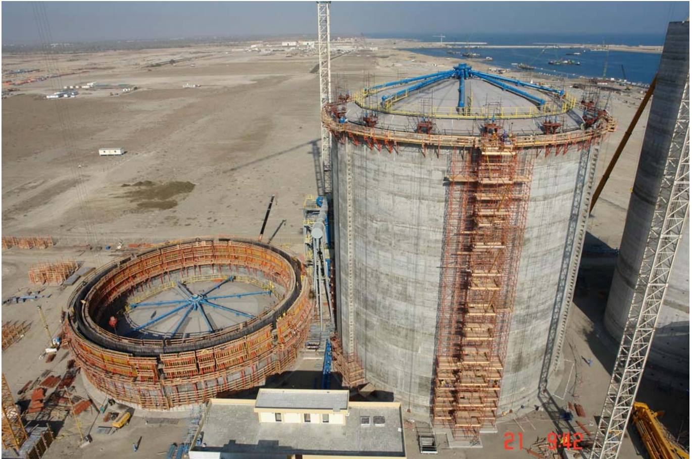
▲ First silo: roof lifted, Second silo: walls under construction and roof still waiting to be lifted!
