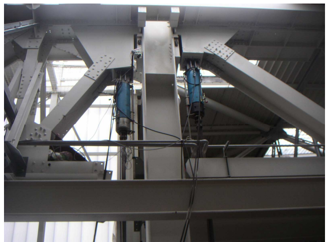
▲ Lifting units in parallel connection – installed under the roof upside down
