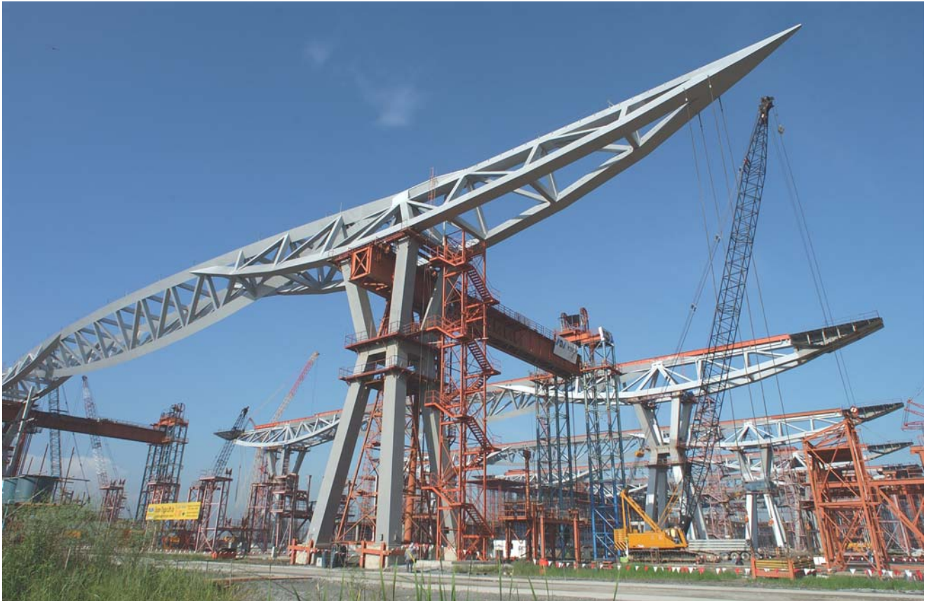
▲ Lifting Super Truss, with previously erected Super Trusses in the back ground
