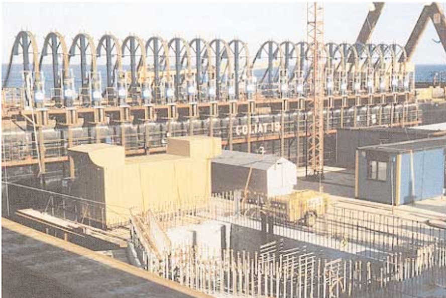
▲ Lowering operation with 20 VSL strand lifting / lowering units SMU-330 on each barge.
