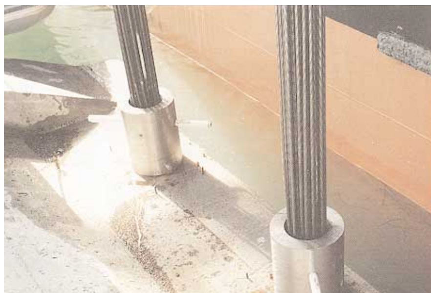
▲ Screw-type couplers connected each strand bundle with a stressing head of the vertical VSL caisson post-tensioning cables. Thread size and thread tolerance as well as greasing
