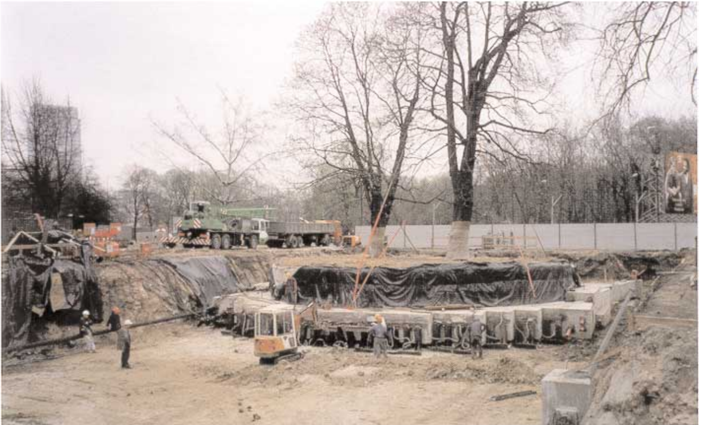
▲ Sliding of tree 32 and 33 in the Saski Business Park
