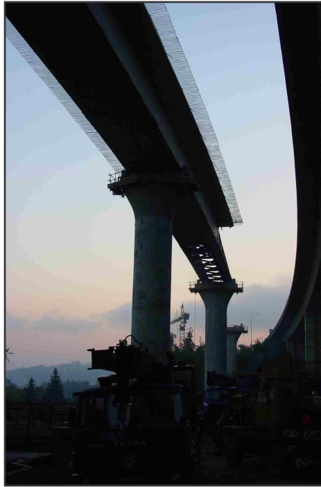
▲ Top slab cantilevers will be poured after launching finishing and precast wings installation.
