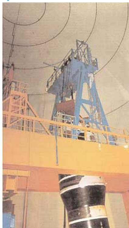
▼ Lifting gantry on polar crane.
